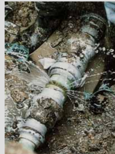
Water from Gas Pipe
