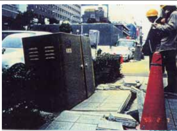
Damage to underground lines
