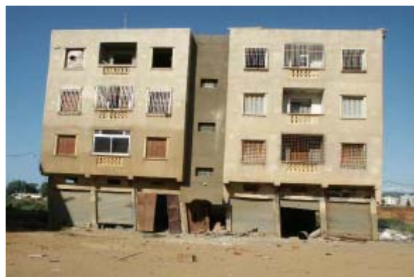
Figure 9. Example of 4-story building (shown by red circle in Fig. 8-a and -b) suffered from soft story damage corresponding to Grade 4, was incorrectly judged as Grade 1-2 through visual detection from QuickBird images.
