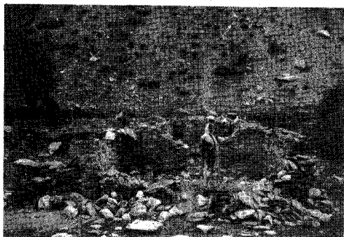
Photo 1 Collapsed dry masonry wall
