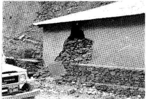
Photo 16 Wall breached by boulder which is still inside this building
