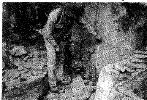
Photo 18 Uneven ground settlement, Barikot
