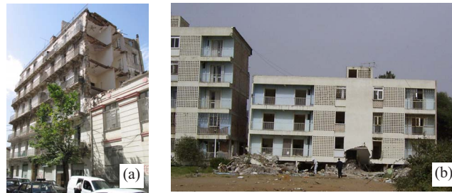
Figure 5. Typical damaged buildings in the area of study. (a) Exterior wall collapse of a 6-storied old masonry building (EMS-98=VI) located in a dense urban area, not far from Hussein-Dey ST. (b) Collapse of the first and second floors of a 5-storied RC building (EMS-98=X) 600 m away from the Boumerdes ST.
