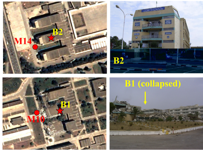
Figure 11. Example of two three-story RC buildings with the same structural characteristics located in two different zones in Boumerdès within approximately 1 km of each other (see Figure 6). B1 is located on the south campus of Boumerdès University, whereas B2 is located on the north campus.
