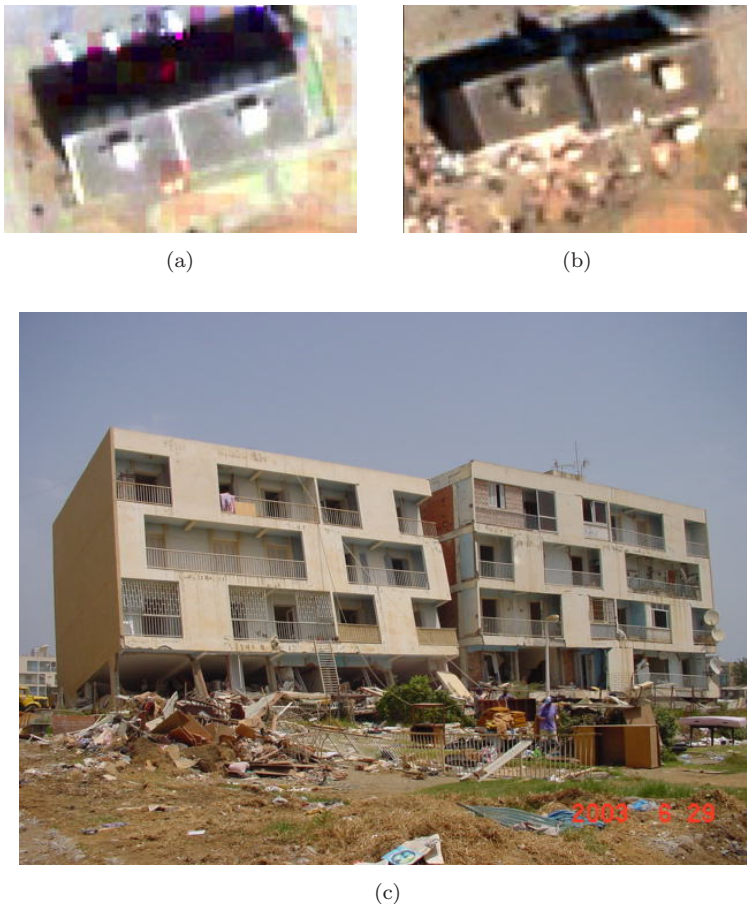
Fig. 11. Damage detection accuracy for a heavily tilted building: (a) the pre-event QuickBird image, (b) the post-event QuickBird image, and (c) a photograph from the ground.
