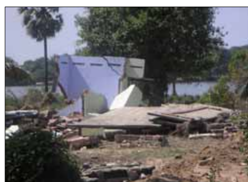
Totally collapsed building
