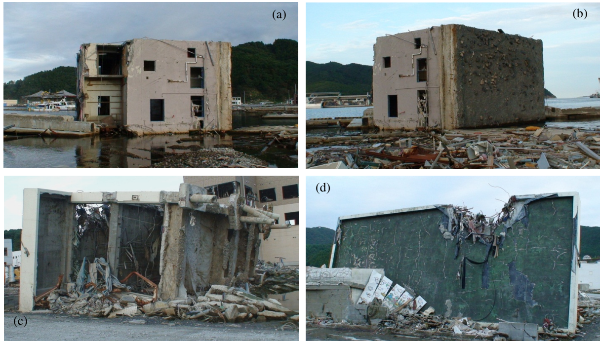
Figure 7: Damages on Reinforced Concrete buildings
