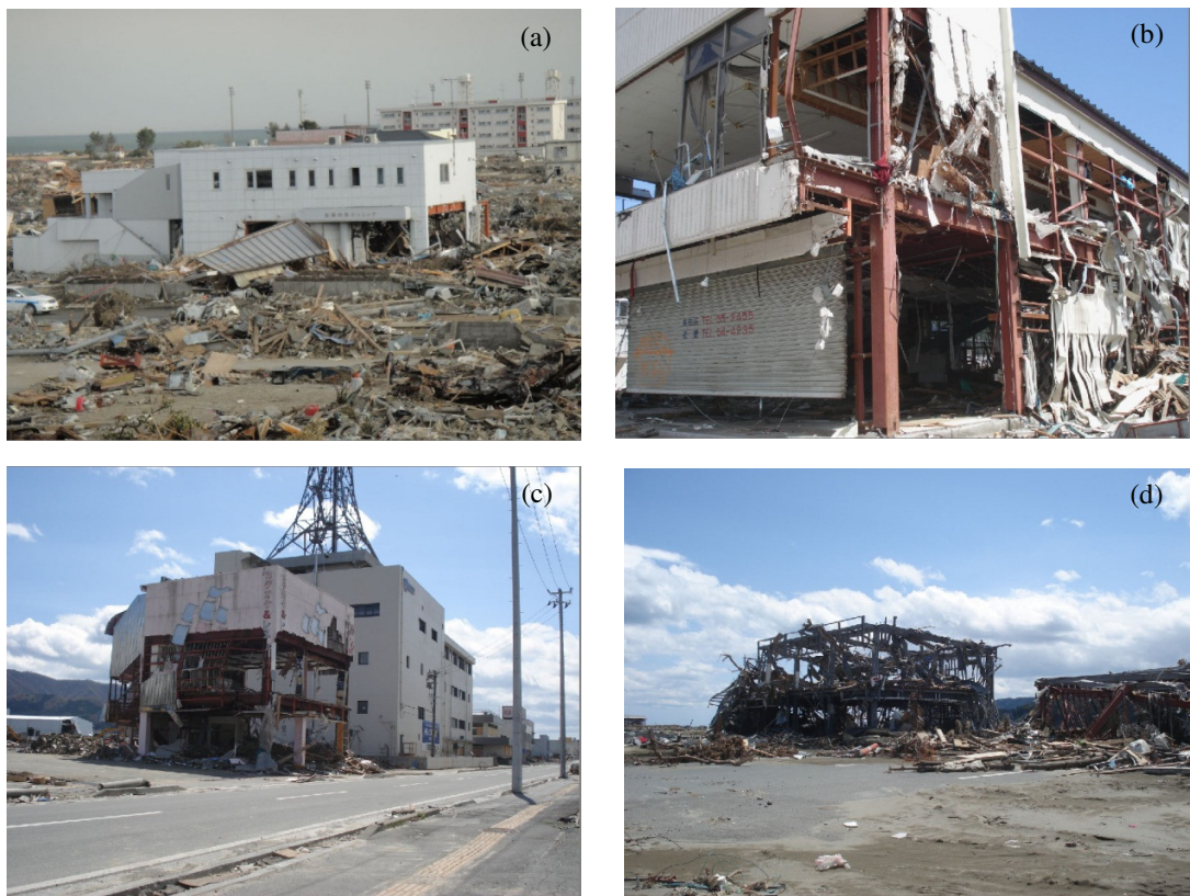
Figure 4: Damages on steel structures
