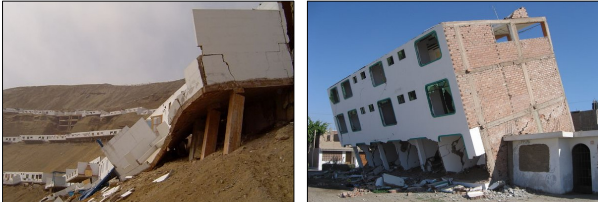
Figure 1, 2: Evidence of excessive displacement on very superficial concrete slab foundation (the design was based on the inertial model and horizontal force of the Peruvian Technical Standard E0.30 for Earthquake Resistant Design, and did not consider the effect of the horizontal and vertical displacements during the earthquake). Earthquake 8.15.07 in Pisco, Peru.
