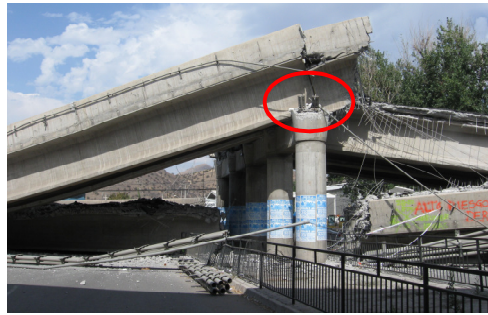
(a) Collapse of eastbound Lo Echevers overpass
