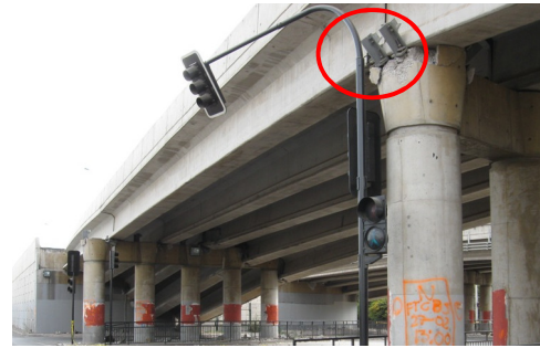
(b) Collapse of eastbound Miraflores overpass
