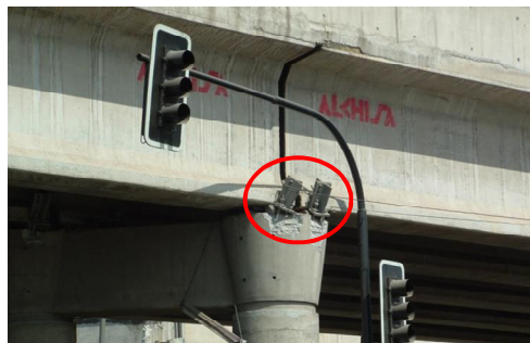
(c) Damage of westbound Lo Echevers overpass
