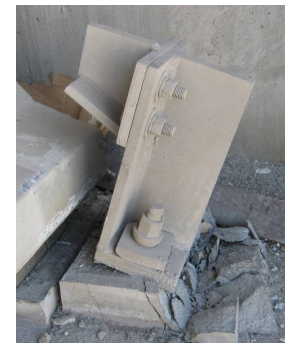
(b) Damaged to steel stopper
