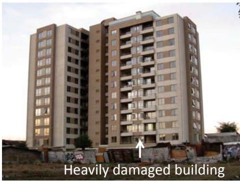
Salas 1343 building Heavily damaged building at Concepción city during the 2010 Maule earthquake
