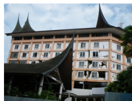
Heavily damaged in 2009
