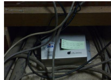
1st Floor: Control room
